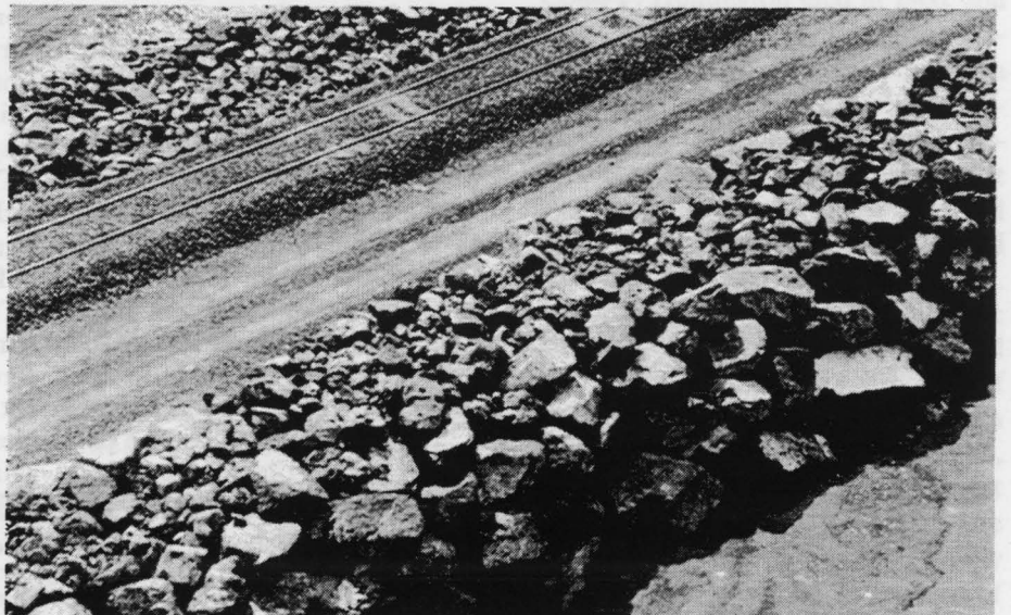
Southern Pacific track showing the three sizes of rock used to protect the fill. Lynn Farrar photo.
