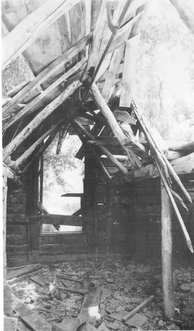
The livery barn's roof has collapsed, but old harness and other tack items still hang from log walls in this nearly a century old structure.
