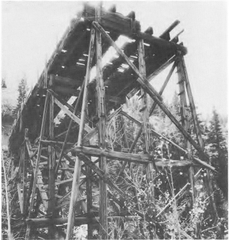
Opposite one of the old mines at Sweet is this large tressle which once carried coal from the mine high on the canyon wall to the tippie below.
