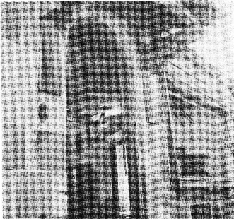
About all that remains of National is a row of tile homes with beautiful arched doorways and large picture windows opening across the canyon.
